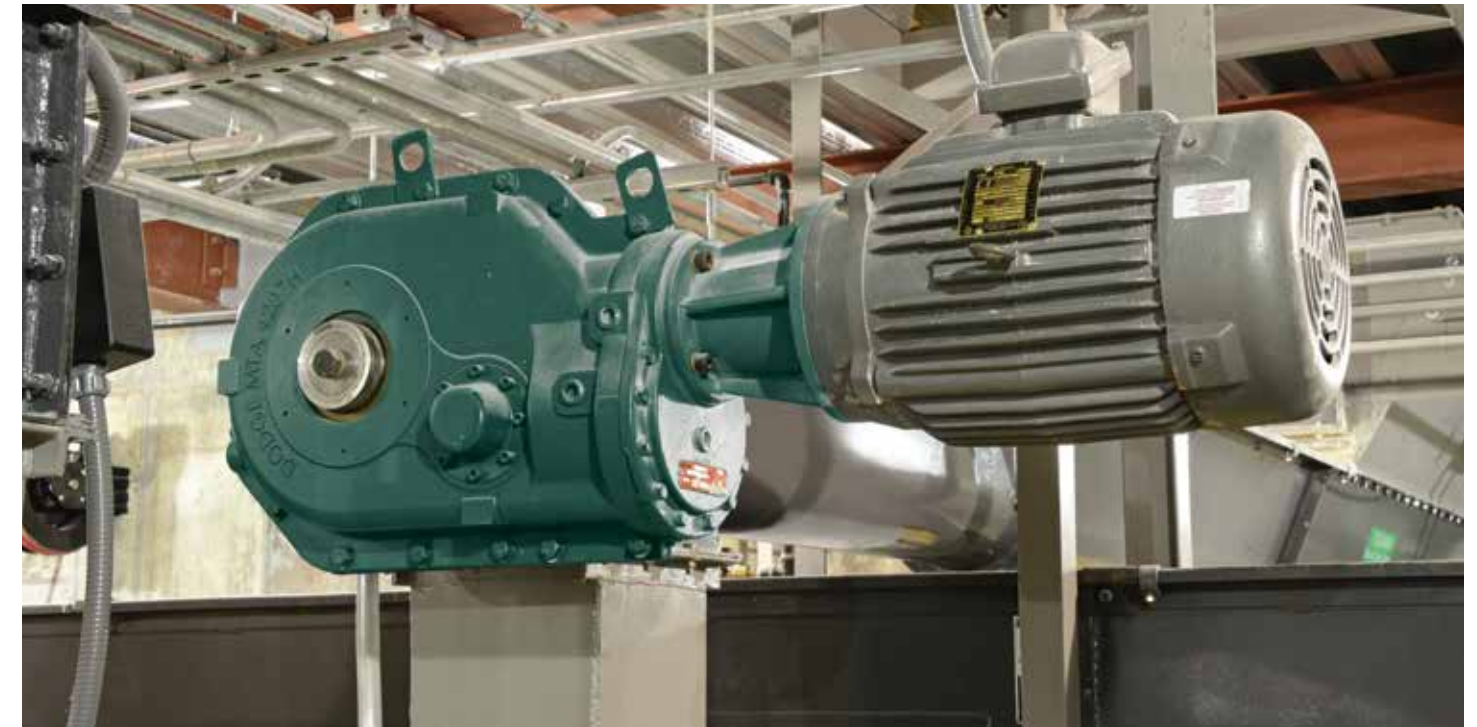
Baldor•Reliance explosion-proof motors and Baldor•Dodge Motorized Torque-Arm II gear reducers were selected for the grain-receiving screw conveyors, which are located in the basement of the building. This explosion-proof motor provides excellent energy savings with its NEMA Premium® efficient electrical design. Full cast iron motor construction with a corrosion-resistant epoxy finish provides long life in this hazardous industrial application. The motor nameplates are clearly marked by UL and CSA for the hazardous environment. The MTA is a right-angle, beltless direct drive solution that features a patented sealing and drive shaft system, resulting in reduced maintenance requirements.
