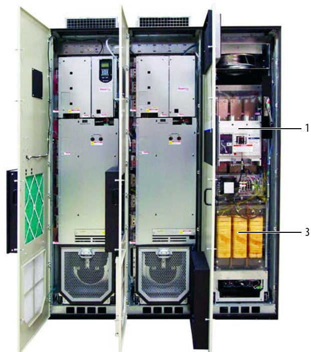
Input power landed behind circuit breaker, which is accessed by extracting rollout chassis.
